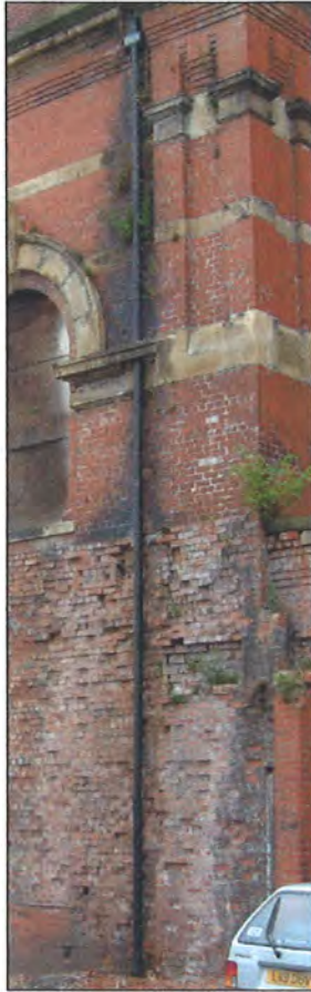
Plate 13: Example of Brickwork being Damaged by Poorly Maintained Rainwater Down-Pipe
