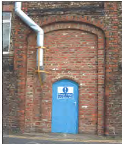
Plate 9: Example of Bricking-Up of an Original Opening in External Wall to Suit New Use of Building
