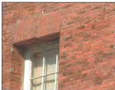
Plate 6: Example of Brickwork Lintel where Bricks have Slipped but Currently Awaiting Repair
