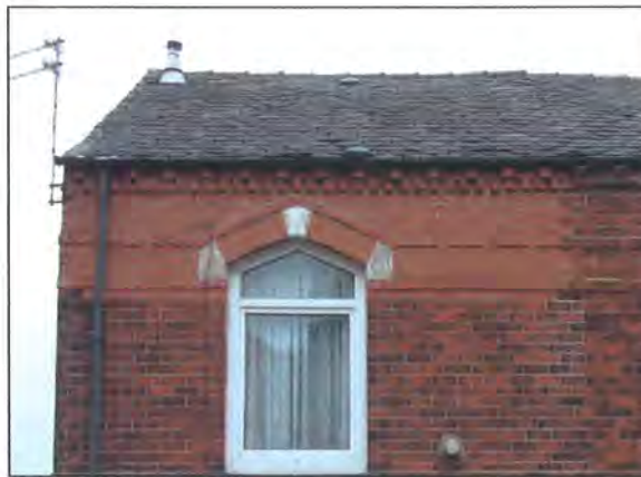
Plate 8: Example of a Brickwork Lintel that was Repaired Using New Bricks (Note: The brickwork over lintel was also replaced)
