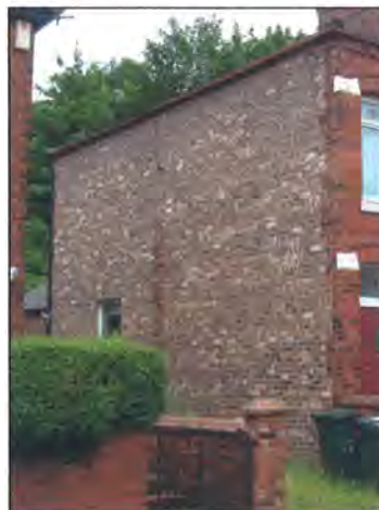
Plate 16: 1930's End Terraced House Where Whole Gable Wall Was Recently Rebuilt with New Brickwork
