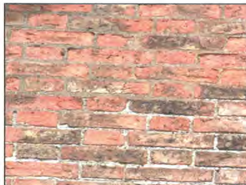
Plate 12: Example of Spalled Brickwork
