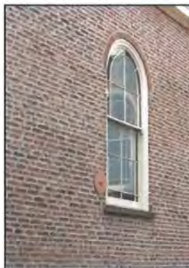
Plate 10: Example of Steel Tie Rod Inserted Through Building to Control Bulging in External Wall
