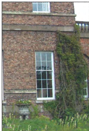
Plate 14: Example of Managed Growth of Vegetation on External Brickwork Wall
