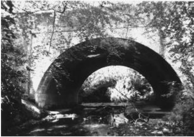
Figure 4 - Elevation of Cascade Bridge, age 175-years. The structure has a clear span of 10.5m and a width of approximately 12.5m. The bridge is entirely of brick construction apart from a concrete slab footpath on one side. The structure provides for a single lane carriageway of width 9.5m and spans a small stream with large seasonal flow differences.
