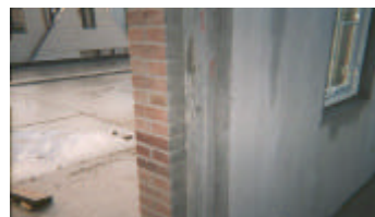
Figure 6 House panel interface detail Courtesy of Redex Export Consultancy.
